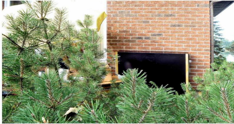
Fig. 4: Air-heat exchanger. The 50 kW air-heat exchanger transfers heat into the ground loop of the test-bed system
