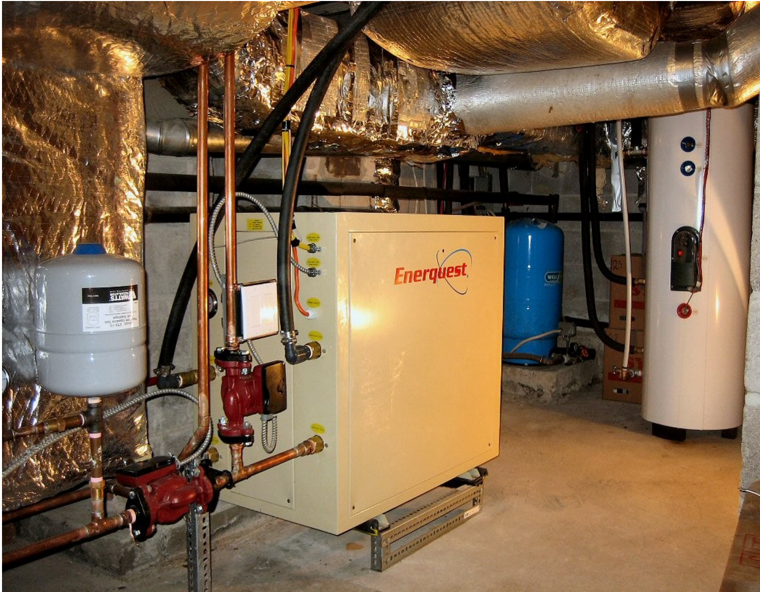
The heat pump provides both underfloor and forced air heating
