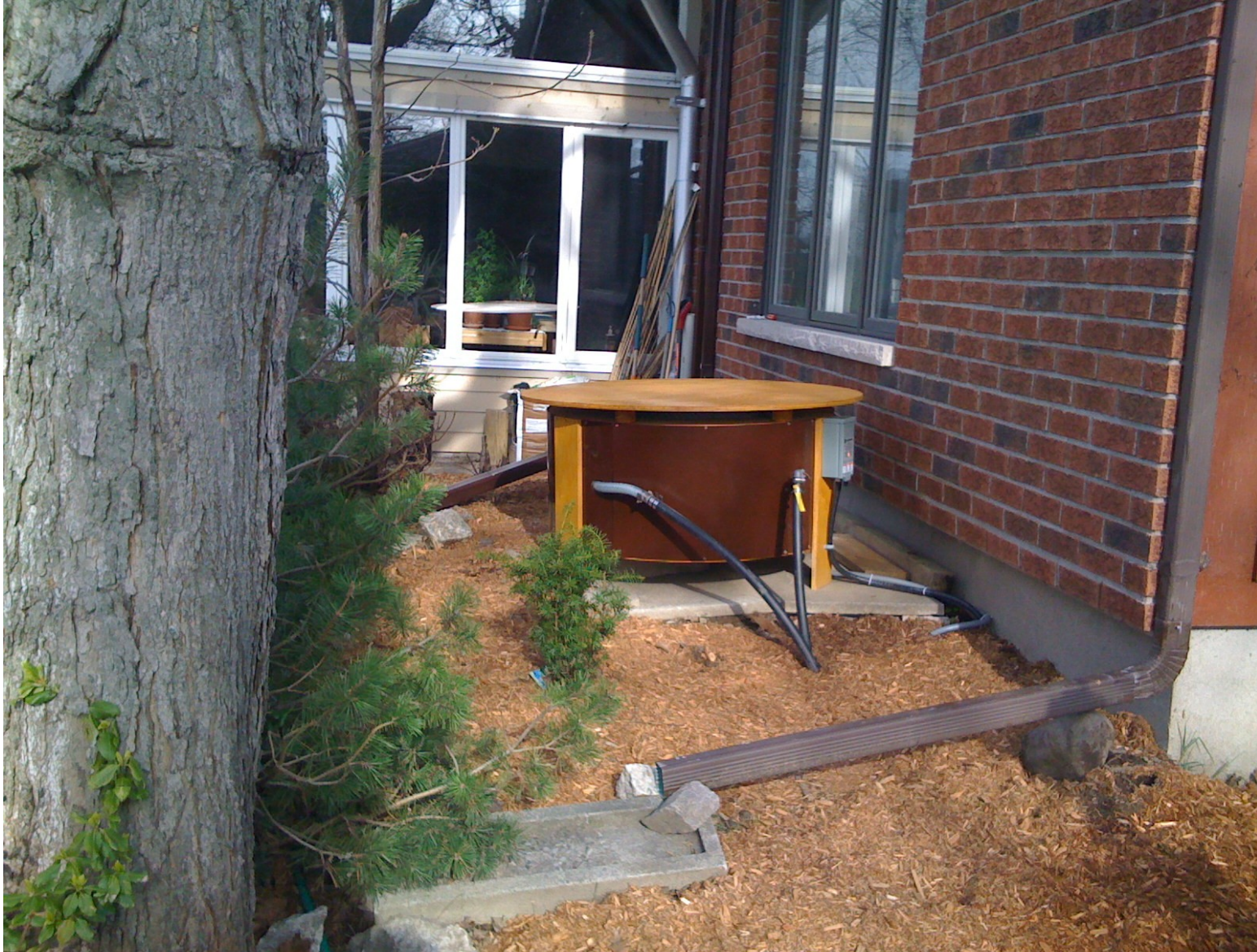
Heat injector box
