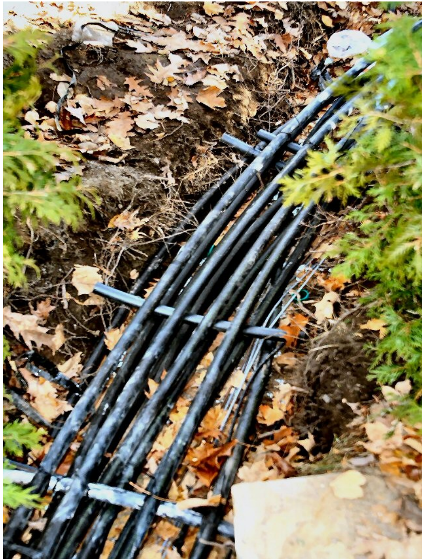
Tubes from the six boreholes lead to the house
